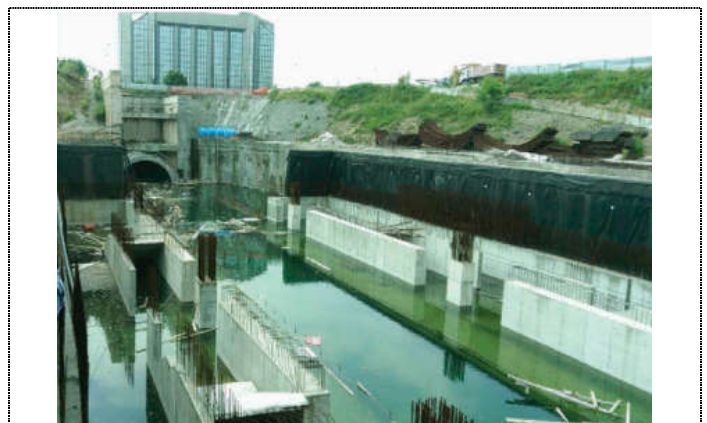
Figure 4. Flooding of the executed works
