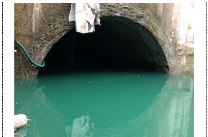
Figure 3. Flooding of the executed works
